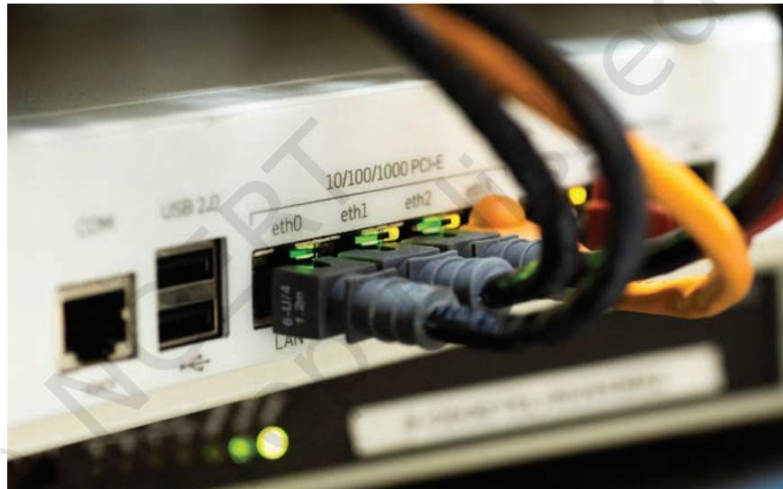
Figure 5.9: Cables connected to a network switch
