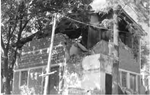
Figure 6.1 : A Damaged Building Due to an Earthquake
